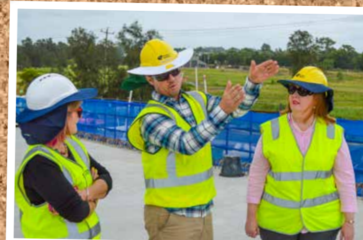
MAITLAND OVERPASS – taking a look at the construction of the Maitland overpass.
